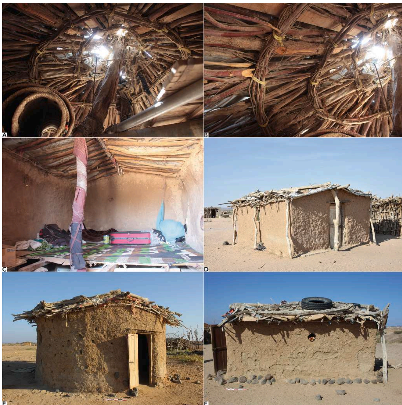
Fig. 7. Roof shape and framework. The concentric frames of the conical roof are arranged radially and grouped together at the top of the roof (A) attached with plant or plastic ties (B). For the gable roofs, the ridge pole is made of a metal tube while the purlins are made of wooden logs and attached by plant ties or pieces of fabric (C). The slope of these roofs is gentle and reinforced by posts placed at the corners and on the lengths of the building on the outside (D). The framework is covered with mixed materials including plastic tarpaulins, textiles, concrete blocks, and even tires (E-F) – Copyrights: Q. Aubourg, E. Baudouin.
