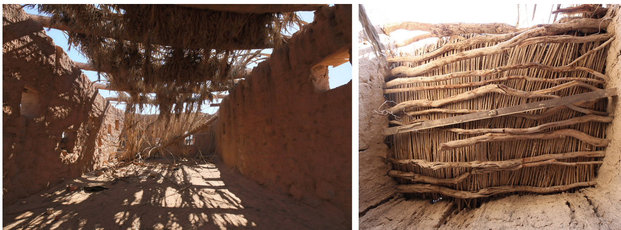
Fig. 8. Examples of roofs using beams made of palm tree (left) and acacia branches (right). © E. Laroze.
