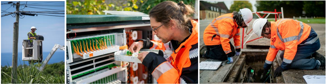
Figure III-3- Telephone pole (left), network cabinet (middle) and underground chamber and its trapdoor (right)
