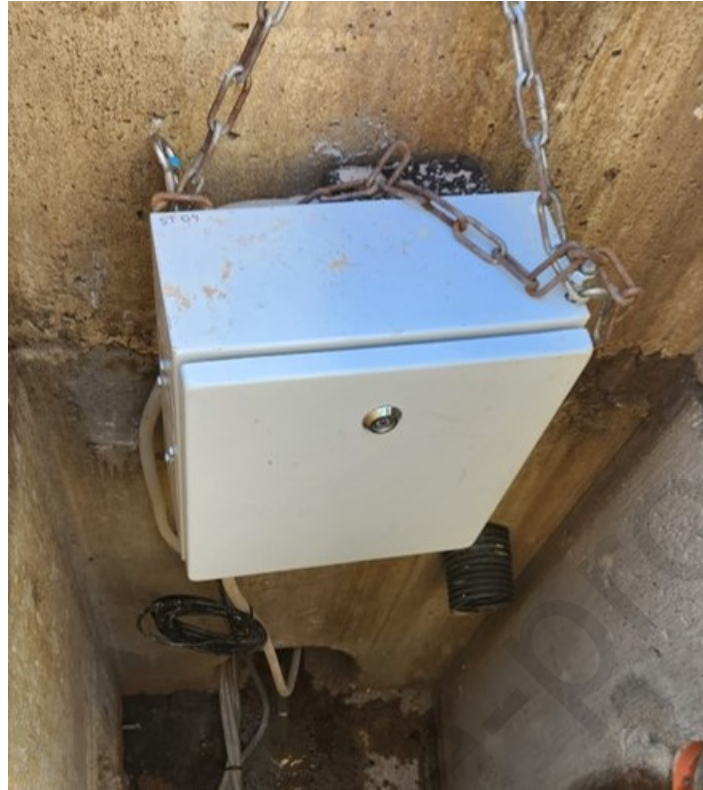
Figure 9 - Monitored station suspended by chains on a wall inside a stormwater drain.
