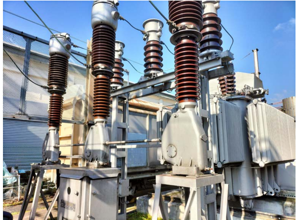
AC circuit breaker at SNCF Railway Test Agency (AEF) traction substation
