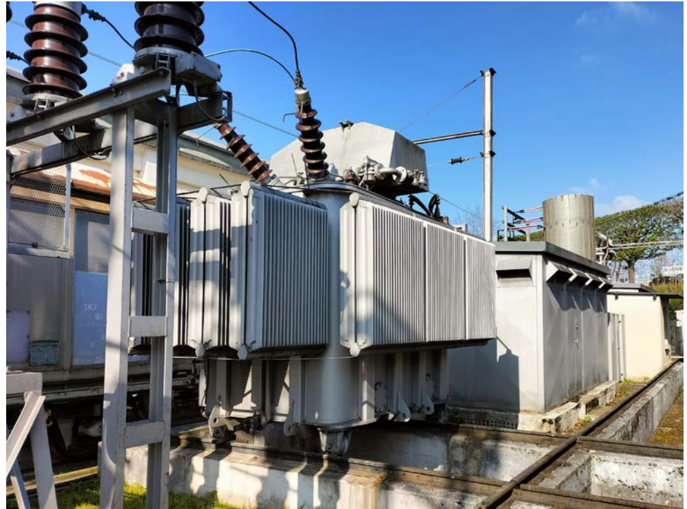
Transformer at SNCF Railway Test Agency (AEF) substation
