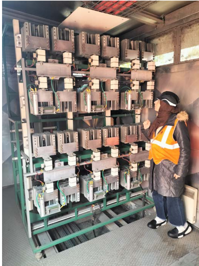
Rectifier C3.P (one half) 6.6 MW at SNCF Railway Test Agency (AEF) traction substation
