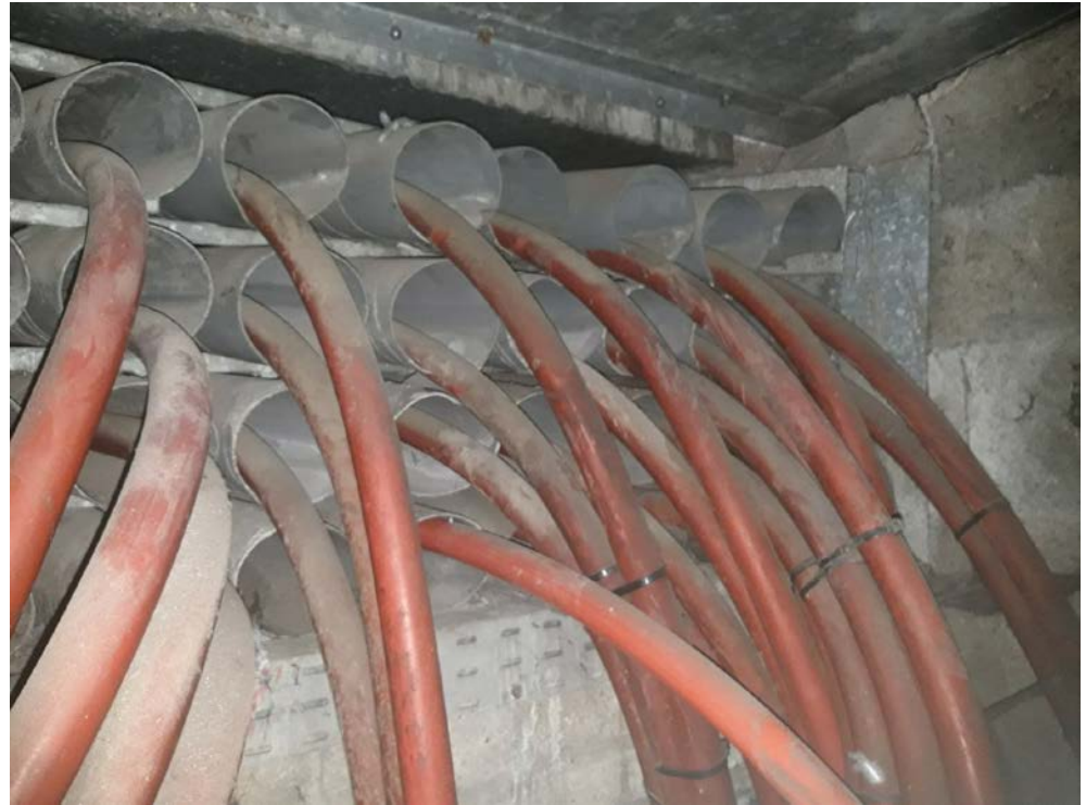
DC power cables at Montparnasse Vouillé traction substation
