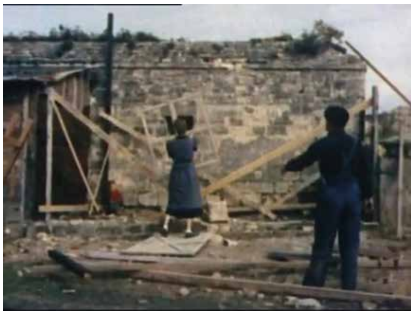
Figure 6.2. Amateur builders trying to build a home on their own. Film still from Somewhere to Live (dir. Jacques Brunius, ECA, 1951).
