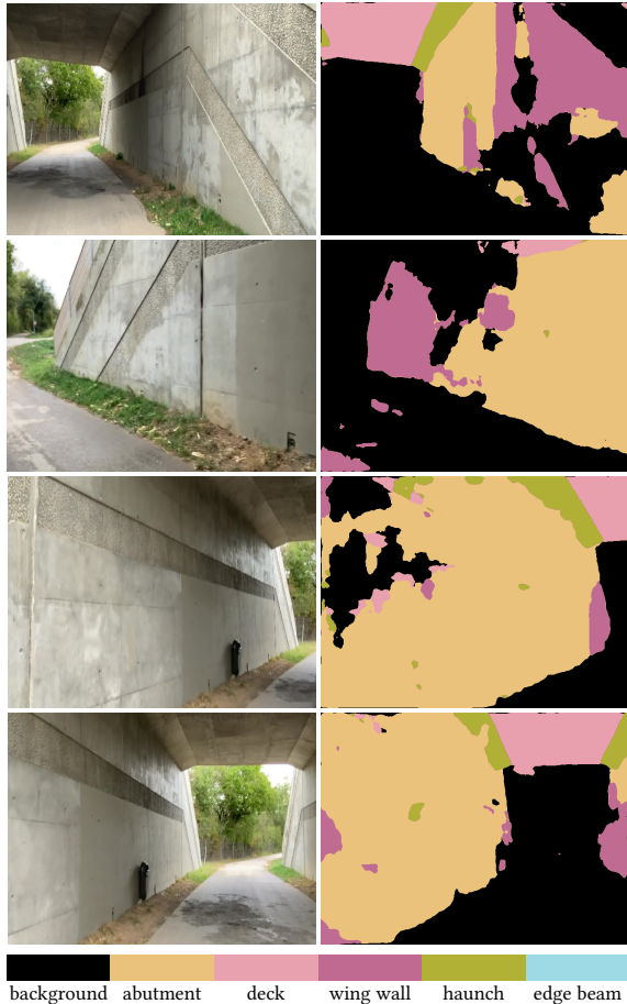
Fig. 12: Example frames of demo bridge on which the annotated point cloud acquisition was tested, along with the per frame semantic predictions during scanning.
