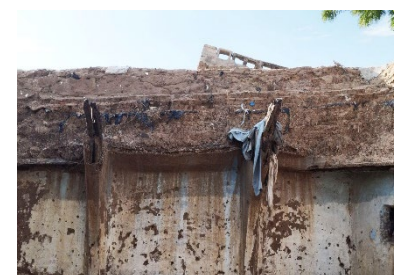
Abandoned earth roof, Bade Community, Gashua, Yobe State - © UniMaid
