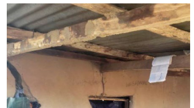
Imported timber suffering from termites, Bama, Borno State - © UniMaid
