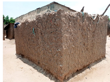
Erosion of the lowest part of the wall. Potiskum, Yobe State - © UniMaid
