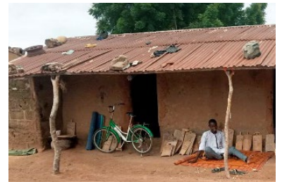
Heavy objects as ballast on top of the roof, Wuroahi Community, Adama State - © UniMaid
