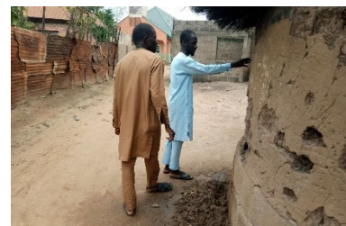
Earth walls requiring re-plastering maintenance, which is more difficult if the plaster is stabilised, Opalo village, Lamurde, Adamawa State - © UniMaid
