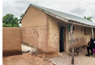
Cement slab next to earthen wall causes damage to wall base, Gombi, Adamawa State - © UniMaid
