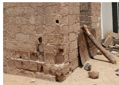
Eroded sandcrete blocks, Pulka, Borno State - © UniMaid
