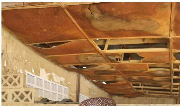
Plywood needing repair, very often because the roof covering is leaking on it, Malakyariri, Borno state - © UniMaid
