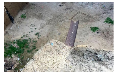
Proper maintenance of the evacuation of an earthen roof, Gashua, Yobe State - © UniMaid
