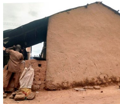
Damaged wall because it lacks of foundations, Wuroahi Community, Fufore, Adamawa State - © UniMaid
