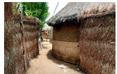
Sandcrete blocks foundation under earthen walls avoids rising humidity, Opalo, Lamurde, Adamawa State - © UniMaid
