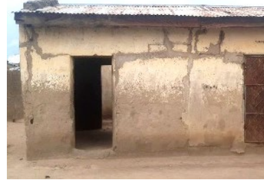
Cracks on sandcrete walls due to the lack of a ringbeam, Bulabulin community, Dikwa, Borno State - © UniMaid
