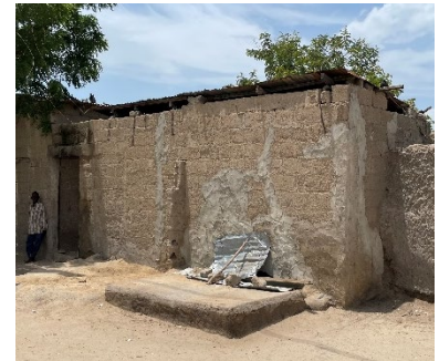
Cracks on sandcrete walls due to proximity to septic tank, Rabiri Community, Dikwa, Borno State - © UniMaid
