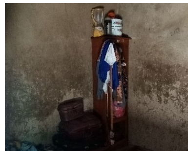
Insufficient indoors light, Bulabulin, Borno State - © UniMaid
