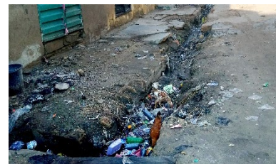
Lack of maintenance of street drainage with cumulation of waste, Bulabulin, Borno State - © UniMaid
