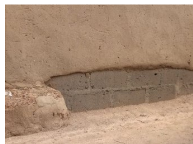
Sandcrete blocks in foundation of an earth wall, Fufore, Adamawa state - © UniMaid
