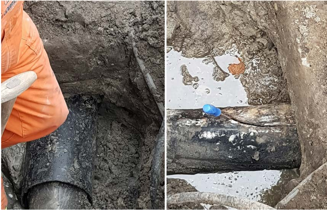
Figure 5.7 A case of poor-quality installation. An external piece of pipe was found to cover a PVC sewer pipe at the point of failure. (Courtesy K. Makris).
