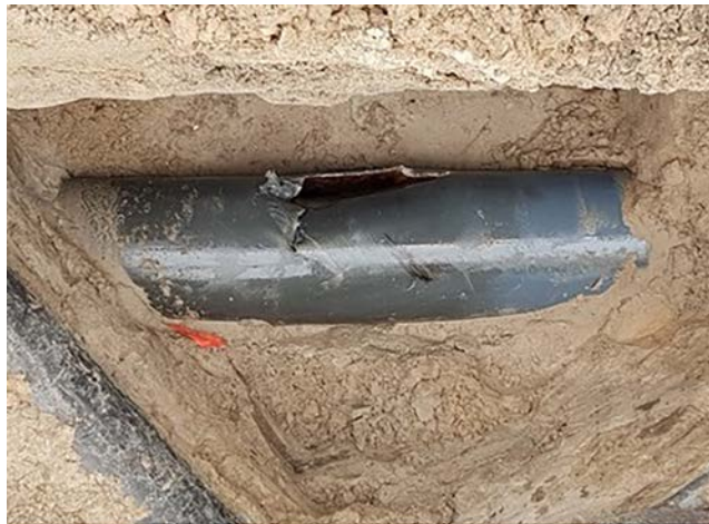
Figure 5.9 A breakage of a PVC sewer pipe due to an external impact (hit by excavator). (Courtesy K. Makris).
