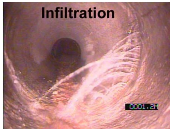
Figure 5.50 Infiltration of groundwater due to a defective joint (Deltares).
