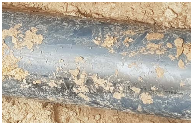
Figure 5.10 PVC pipe with obvious signs of discolouration on the external side. (Courtesy K. Makris).
