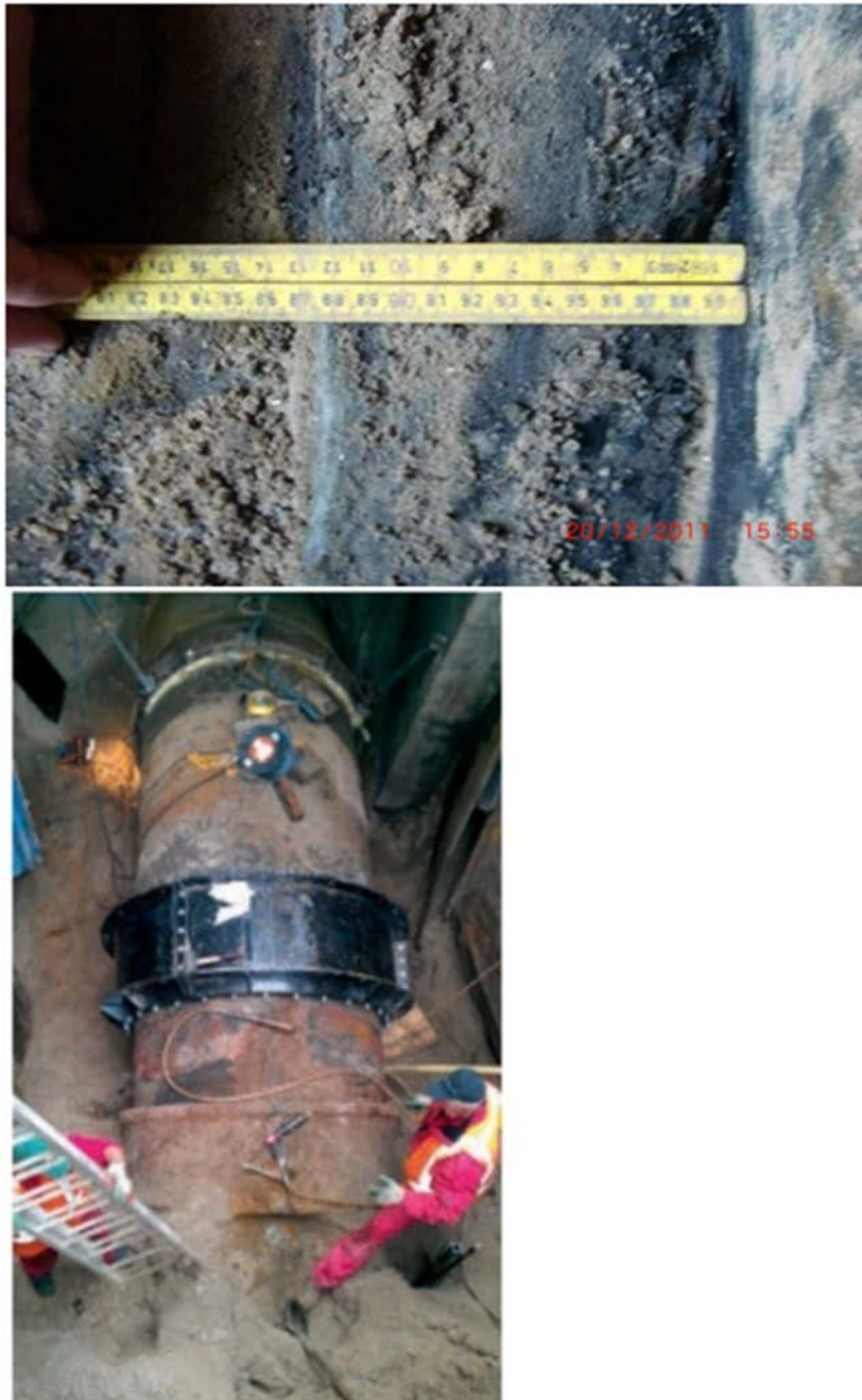
Figure 5.54 Example of a joint that has given way. The pipes were pushed about 13 cm apart leading to a leaking joint. (Photos by C. de Haan).
