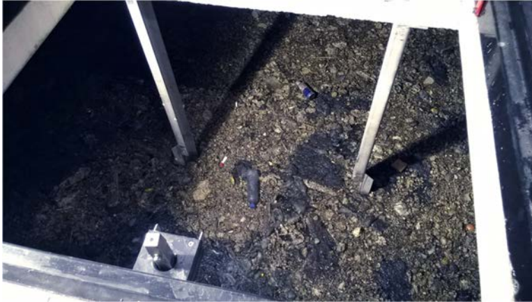
Figure 5.49 FOG in pump well. (Source: Duijnmeijer, 2020).
