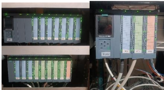
Figure 41: L3 and CSS2 PLC
