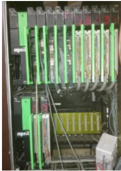
Figure 38: PLC before renovation
