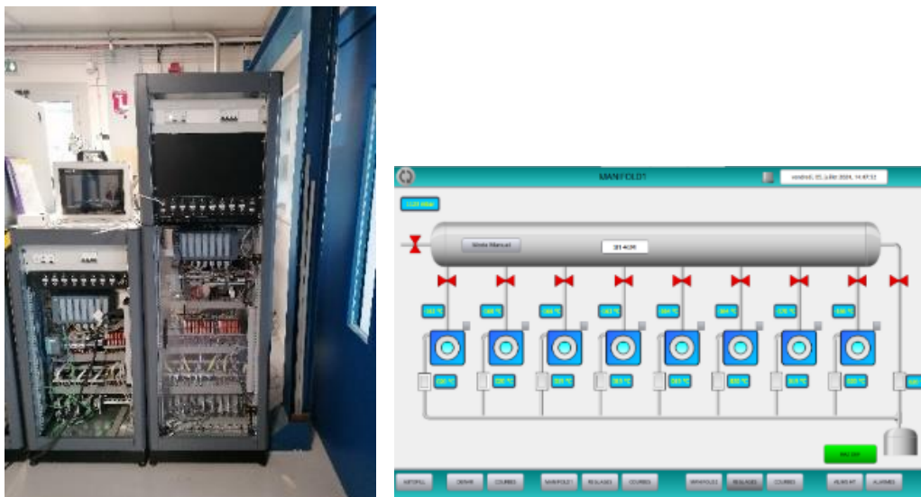
Figure 37: Left :Picture of the new Programmable Logic Controller. Right : Supervision of the Autofill Cabinet
