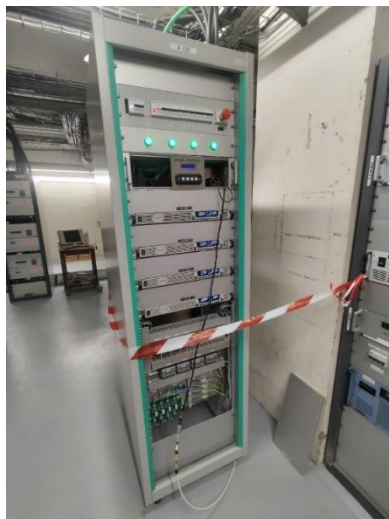
Figure 75: Prototype of power supplies refurbished for magnet
