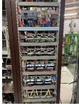
Figure 39: New electrical cabinet
