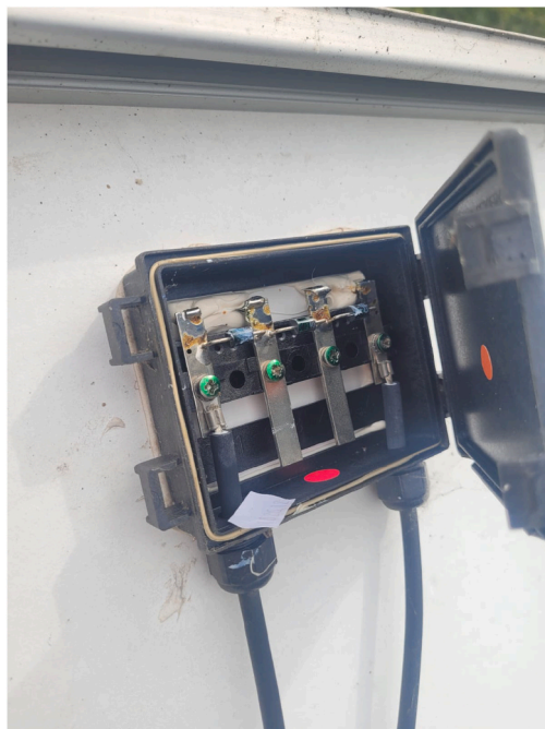
Fig. 3. Bypass Diodes of the PV array.
