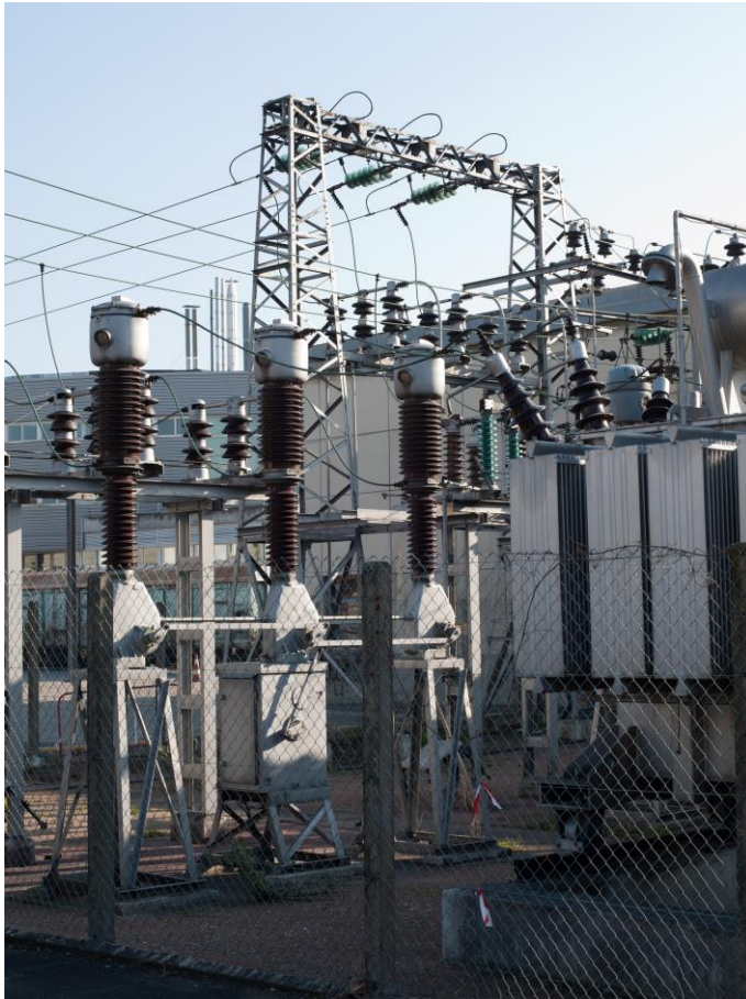
SNCF-AEF Traction substation
