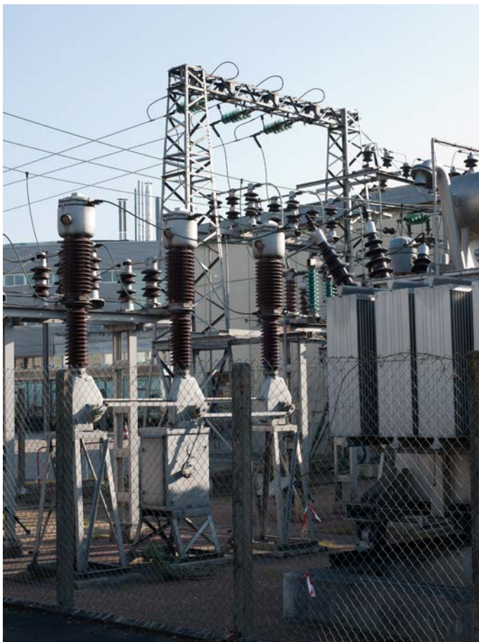
SNCF-AEF Traction substation
