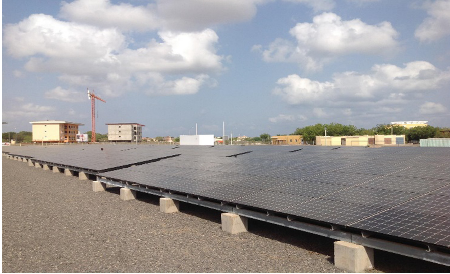
Fig. 2. CERD solar facility.
