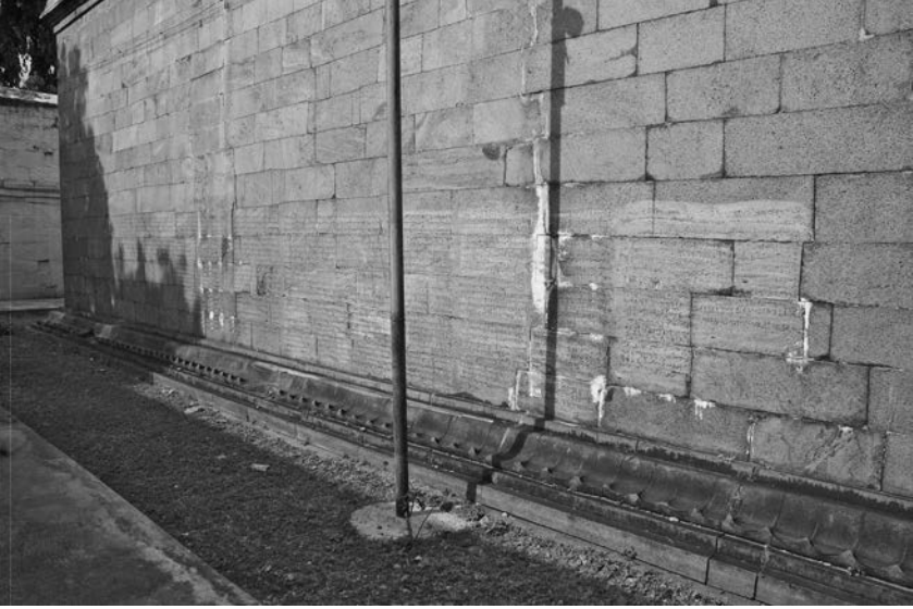
Fig. A.51 Western façade of the compound wall, Tiruvālanturai Mahādeva temple (photo by V. Gillet).
