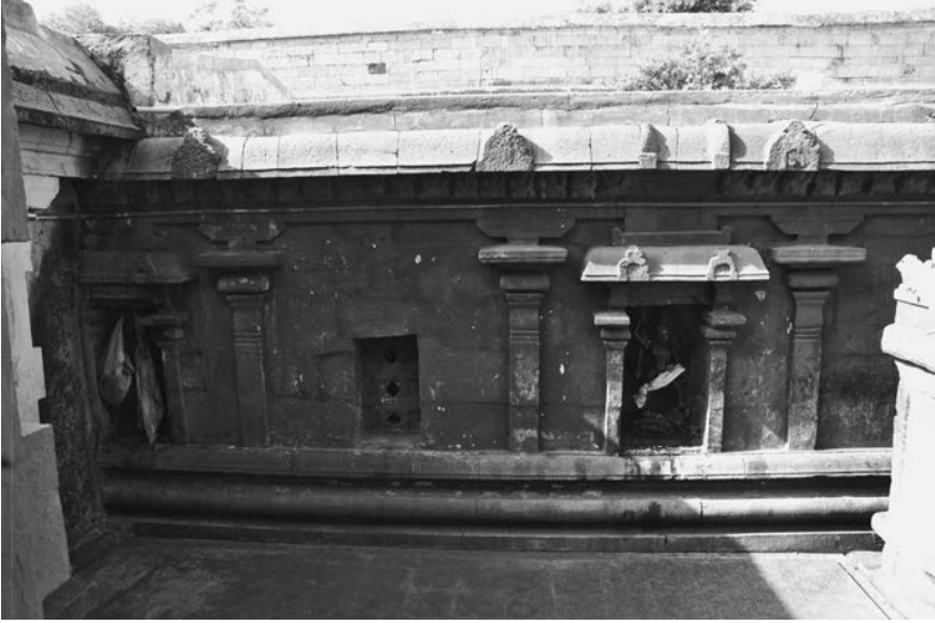
Fig. A.48 Northern façade of the mukha-maṇḍapa of the Tiruvālantūrai Mahādeva temple (photo by V. Gillet).
