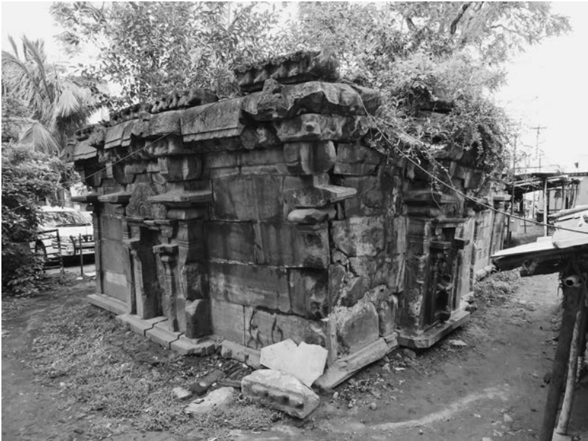
Fig. A.90 Southern and western façades of the Maravanīśvara temple (photo by V. Gillet).
