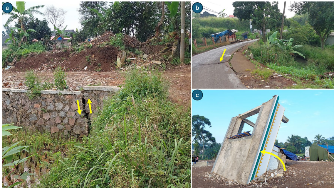
Fig. 9 Field evidence of ground failure due to an earthquake in Cugenang District, Cianjur Regency, West Java: a uplifting and subsidence visible from a dirt road and cracking in a dike, b cracks in the asphalt road indicating soil deformation, c liquefaction resulting in the collapse of buildings (photos taken by Pratiwi)
