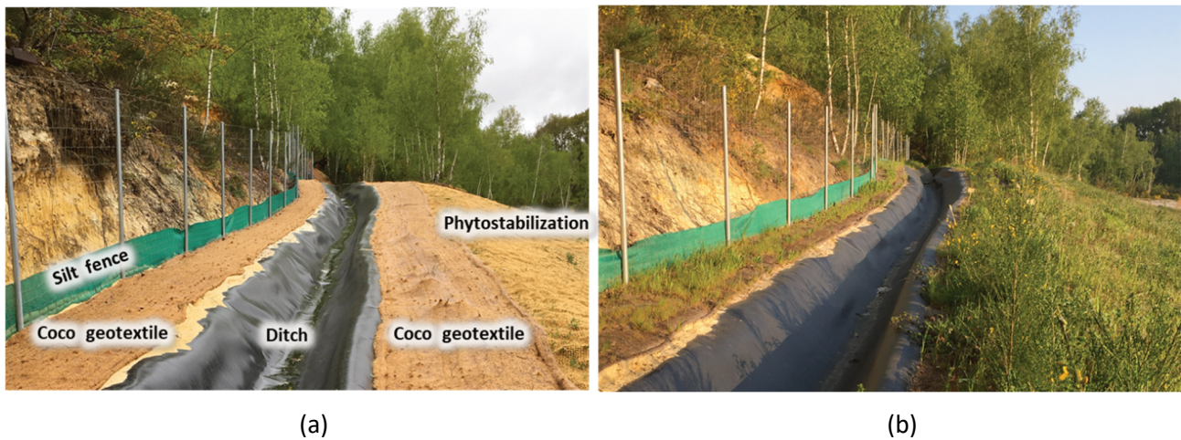
Figure 8 Examples of anti-erosion solutions around upstream rainwater ditches in case study 2: (a) Just after seeding; (b) One year after seeding
