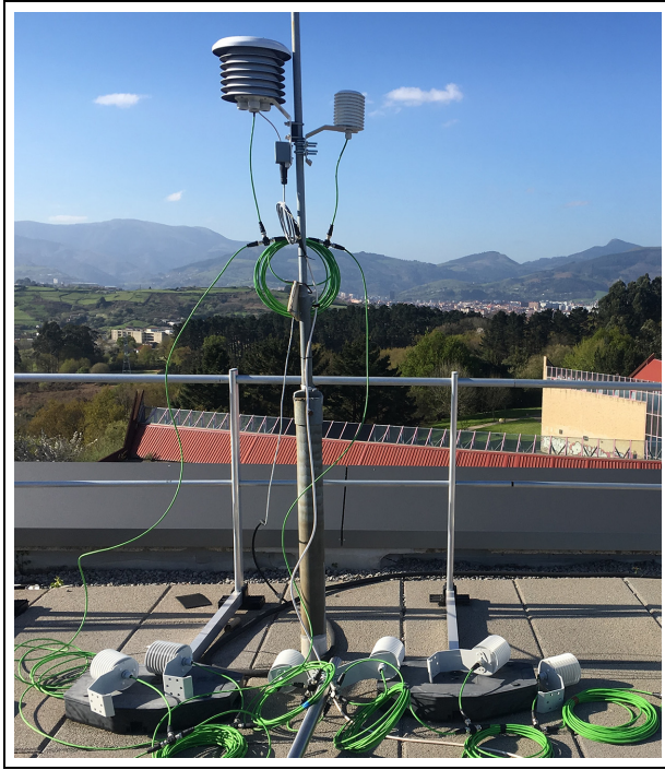
Figure 8. All the shielded sensors for the exterior monitoring system during the installation. The solar radiation shield with mechanical ventilation (on the left) on the mast can be seen together with a solar radiation shield without mechanical ventilation (on the right); these two sensors are already in their final position. Based on Giraldo-Soto et al. (2020).
