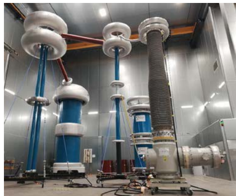
Fig. 3: Experimental setup for the connection of the breakdown test rig (front right) to an AC transformer.
