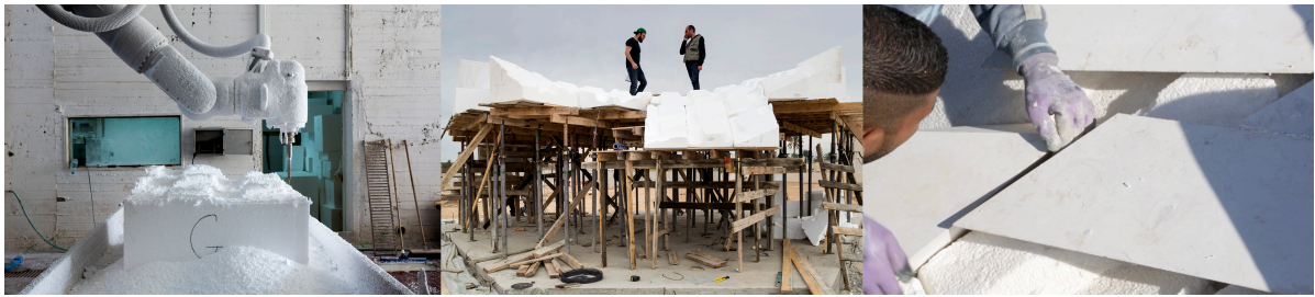
Figure 22: (left) polystyrene blocks carved. (center) timber formwork and polystyrene blocks. (right) placing of stone voussoirs
