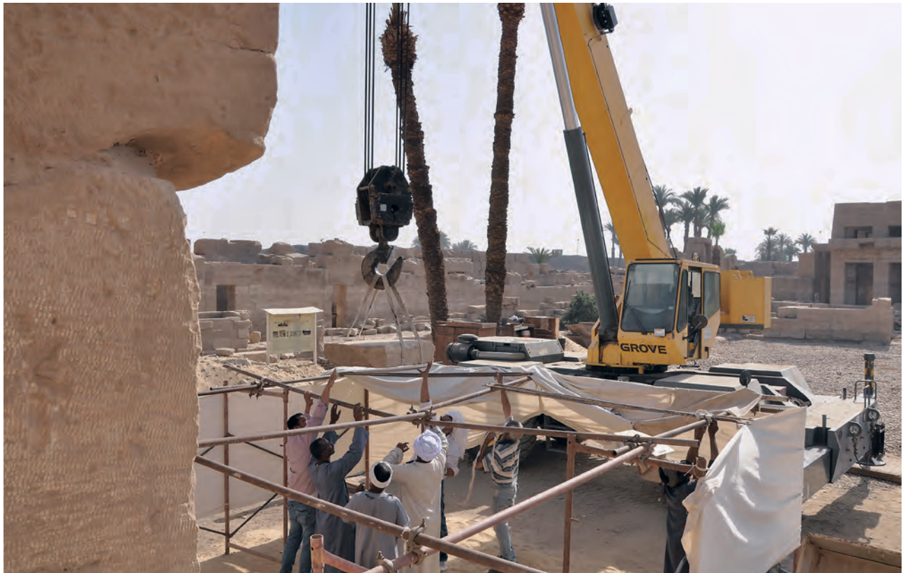
Fig. 5. Removal of the blocks by mean of a crane (E. Saubestre © CNRS - CFEETK).
