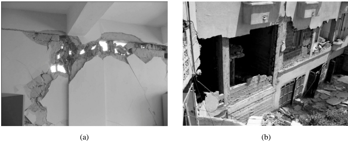
Fig. 1 -Seismic damage in reinforced concrete infilled frames : Bingöl earthquake, Bingöl 2003 [12] (a) and Boumerdes earthquake, Boumerdes 2003 [13] (b)
