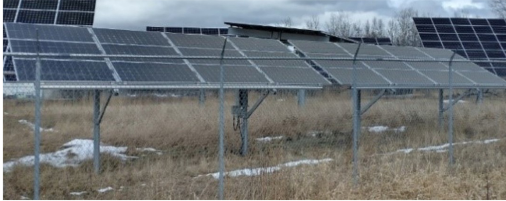
(a) Installed PV Array on the UdeS Campus
