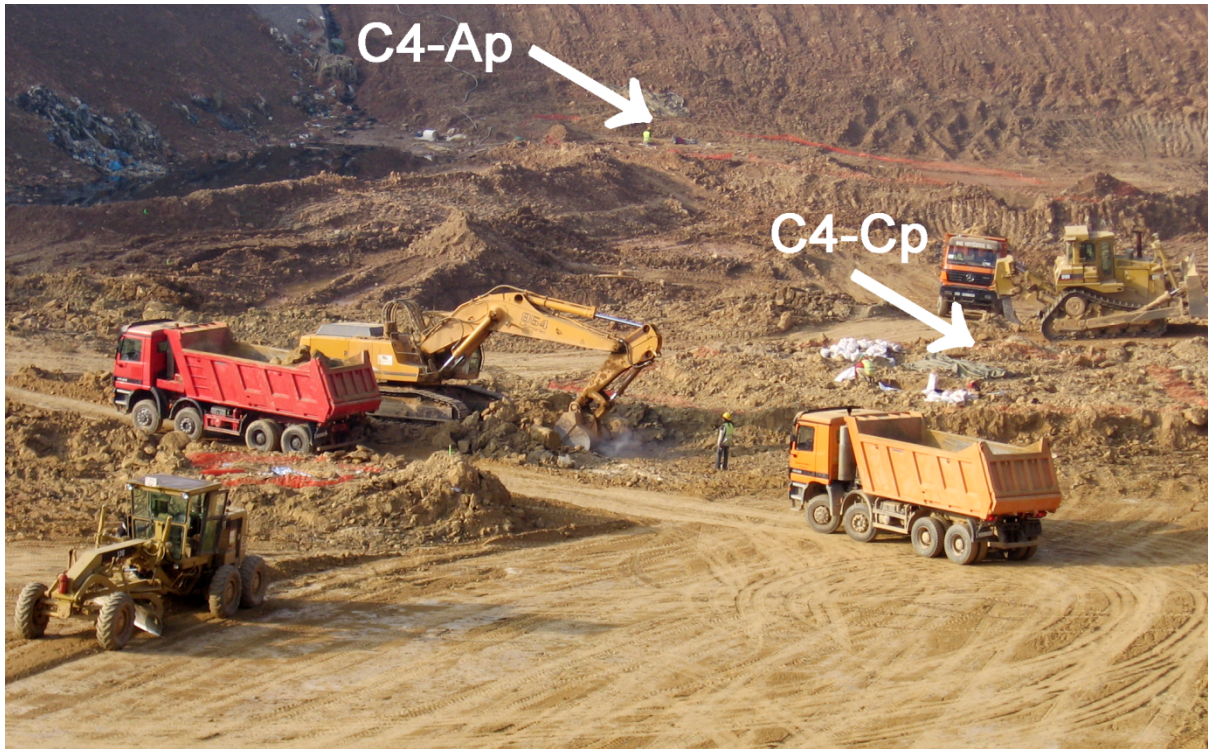
SOM Figure S1. Photograph of the construction of the Can Mata landfill and associated paleontological fieldwork in February 2006, showing the location of localities ACM/C4-Cp and C4-Ap. Photograph © Institut Català de Paleontologia Miquel Crusafont.
