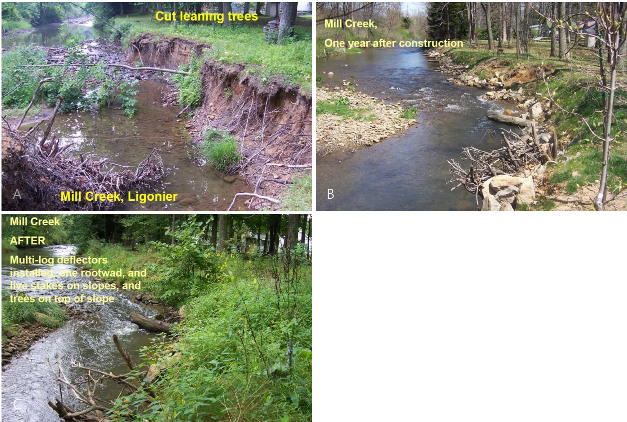
Figure 23. Photos of a fast-flowing river bend where a combination of root wads, log deflectors and live stakes were used for bank stabilisation: (A) before work, (B) just after the end of stabilisation work, and (C) 2 years after the work. (Source: Rob Cronauer, Westmoreland Conservation District, 2016).
