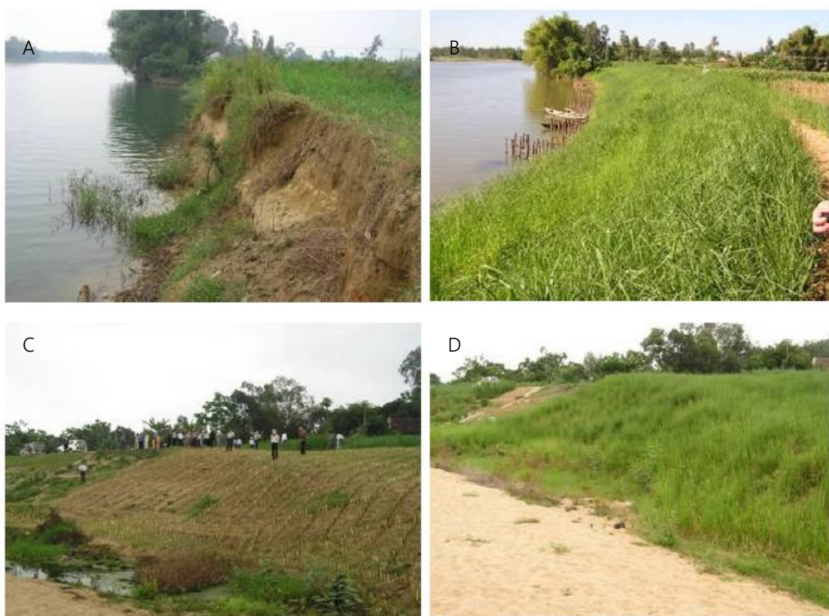
Figure 25. Photographs of riverbank stabilisation using Vetiver in an estuary (A, before & B, after work) and along a large river (C, during & D, after work) (Source: Man et al. , 2011).
