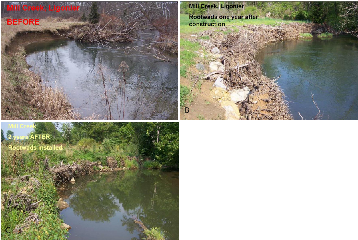
Figure 22. Photos of a river bend where root wads were installed to prevent further erosion: (A) before work, (B) just after the end of stabilisation work, and (C) 2 years after work. (Source: Rob Cronauer, Westmoreland Conservation District, 2016).
