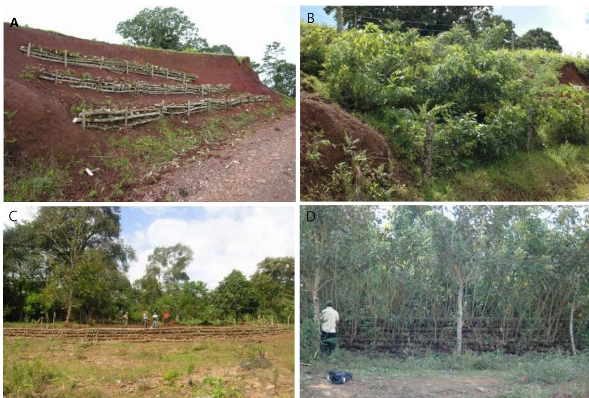
Figure 24. Photographs of the live palisade (A) just after construction and (B) 18 months after construction; and photographs of the crib wall (C) just after and (D) 1 year after construction. (Source: Petrone & Preti, 2010).
