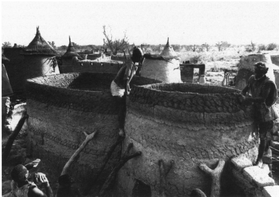
Fig. 3: Two masons on the 'scaffold' place lumps of banco on the upper part of a wall (Esapu, March 1989).
