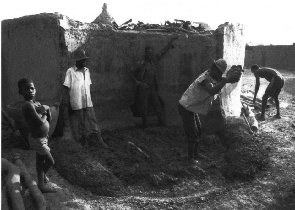
Fig. 5: Laying the base of the wall along the circle on the ground: 'pinning down' the banco (Esapu, March 1989).
