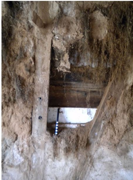
Figure 1. Damaged bousillage construction at the Pigeonnier, Oakland Plantation, Louisiana.
