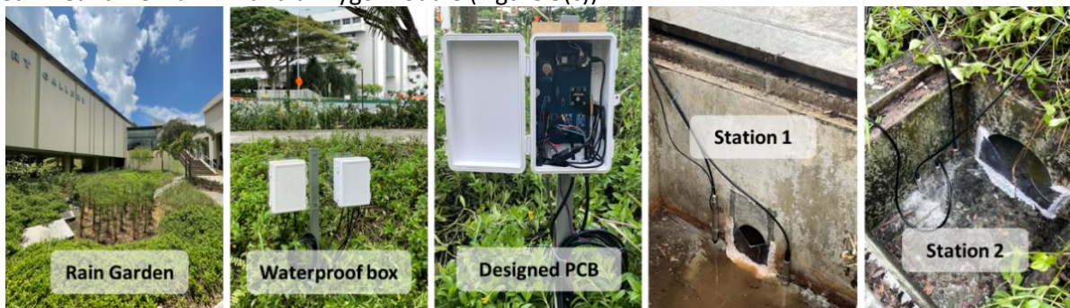
Figure 2. Field implementation of the water level monitoring station 1 and 2 in a Rain Garden in Singapore.
