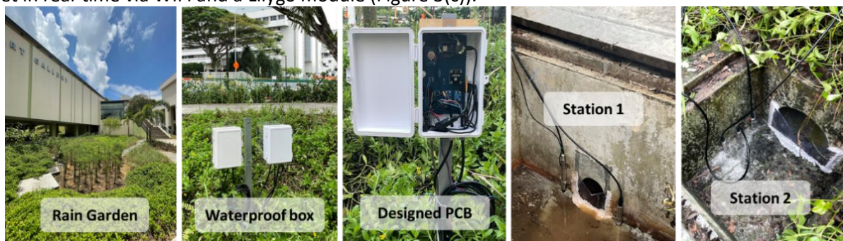
Figure 2. Field implementation of the water level monitoring station 1 and 2 in a Rain Garden in Singapore.
