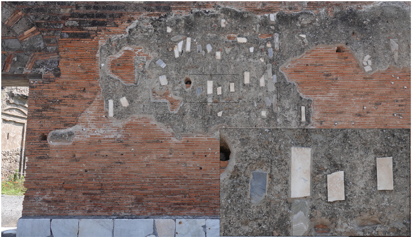
Fig. 10. Front façade of the building known as the “Temple of the Genius of Augustus” (Pompeii, VII 9, 2), with the remains of the plaster for the marble veneers. The marble shims are surrounded by a small void (the two shims on the right side of the zoom) or by restoration mortar (the three shims on the left).
