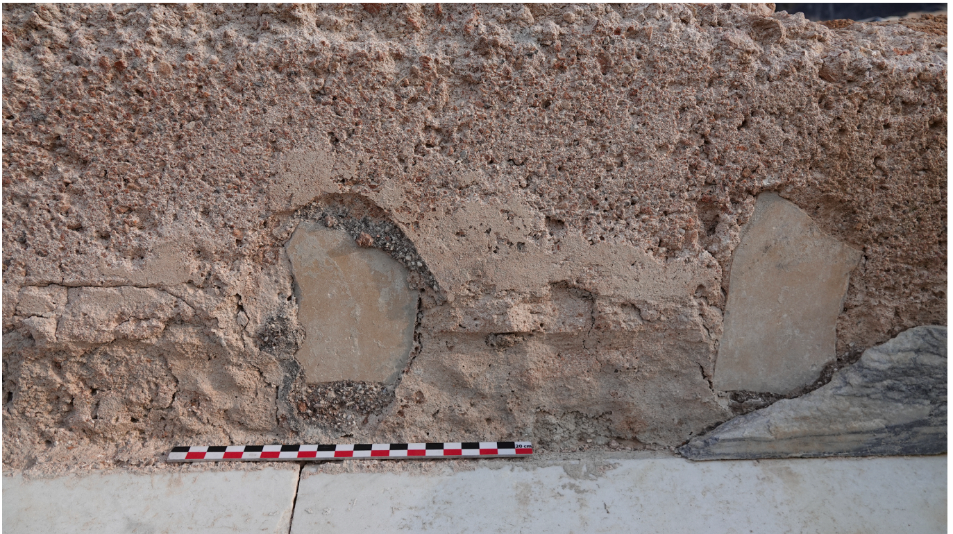
Fig. 3. Detail of the north wall, two shims with all around the remains of a grey and granular mortar.
