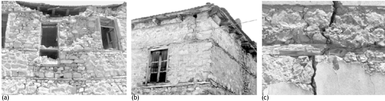
Figure 1a and Figure 1c. Seismic damages on two different buildings in Beltchichta Village (Republic of Macedonia). Figure 1b. Undamaged building in Beltchichta Village (Republic of Macedonia). Credits: M. Hofmann.
