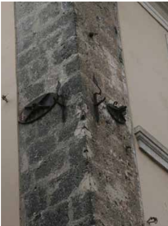
Figure 19: two different types of tie rods on a 15th century building's angle (POURSOULIS, 2009a)
