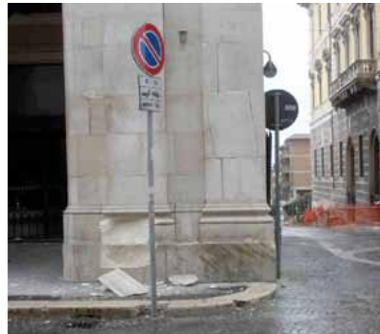
Figure 18b : wreck mechanism of composed flexion on a pillar in 2009 earthquake in L'Aquila (POURSOULIS, 2009a)
