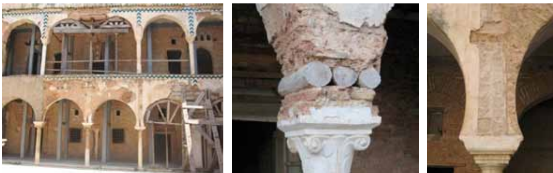
(a) (b) (c) Figure 6: (a) Porch of Dey Palace, Algiers (Algeria); isolator above the capital (b) and at the haunches (c)
