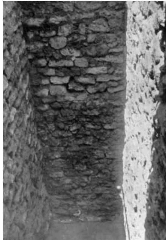
Figure 7b : 7m depth built well for north wing foundation at Knossos palace (EVANS, 1928)
