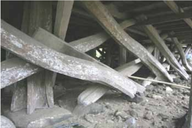
Figure 13: Diagonal bracing in North Nias, Sihare'ö Siwahili
