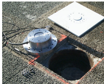
Fig: Excavation in the roadway, sensor, and interface plate (asphalt layer of the wearing course not visible)
