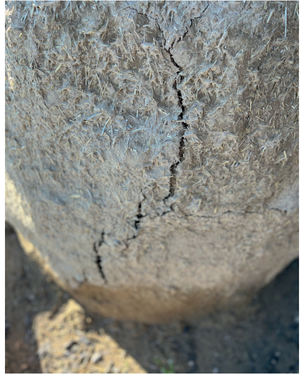
Figure 11. January 2022, cracks in the second silo prototype wall. © Aurélie Feuillas.
