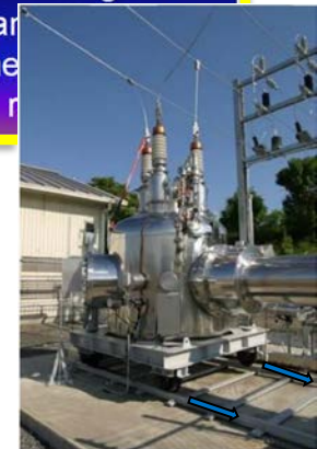
Rollers along the termination for Albany project
