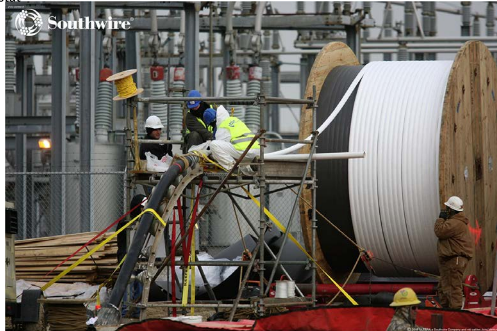
HTS coaxial cable installation for the AEP Bixby project. The white cable on the drum is the superconductor and dielectric portion being fed into the black cryostat and outer jacket.
