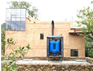
Figure 1. The RWH system of Isla Urbana (Photo: Courtesy of ©Isla Urbana)
