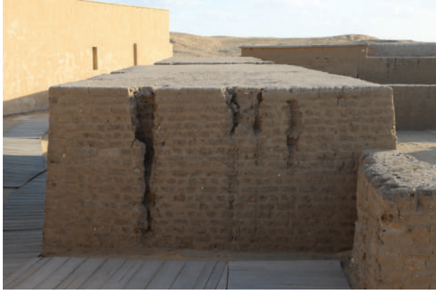
Figure 8: Gullies formed on a recently partially reconstructed entry pylon of one of the tombs of the New Kingdom necropolis at Saqqara.
