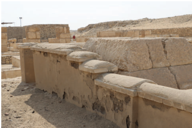
Figure 6: The conservation works (method C) did not prove efficient during the 2020 rains.
