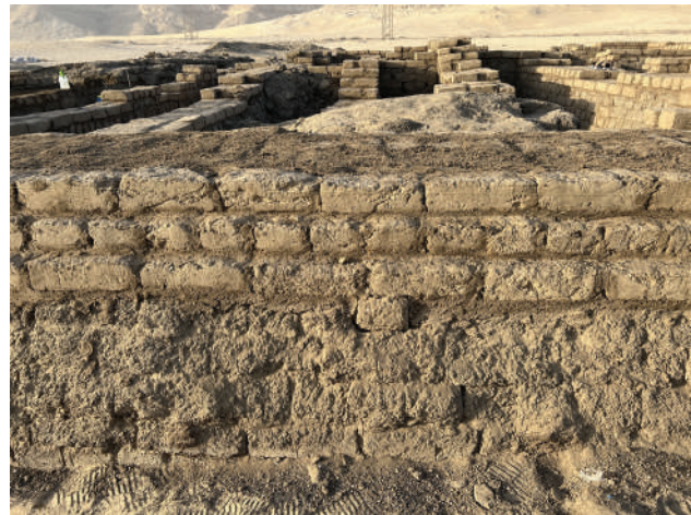
Figure 9: A typical example of an original mud brick wall with courses of new mud bricks, some of which have been textured.
