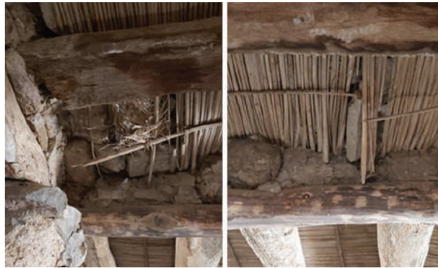
Figure 5: Damaged roofing in room 15.
