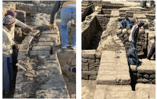
Figure 3: Two deformed walls stabilized with the existing characteristics. © A. Crosby
