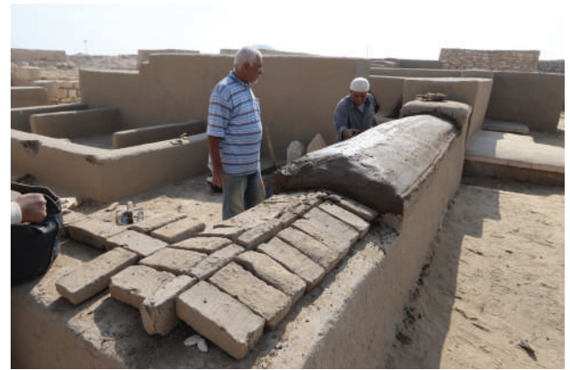
Figure 9: Rounded shape forming the protective capping prepared with bricks and two coats of plaster finish.
