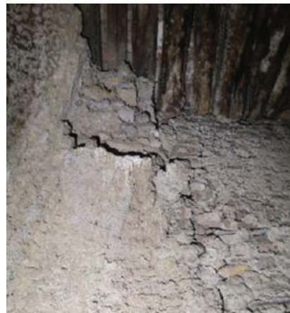
Figure 2: Room 1 western wall - visible cracks. © K. Wasilewski
