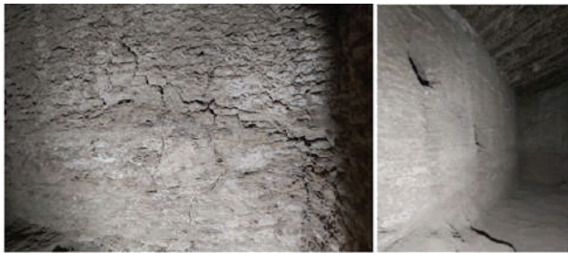
Figure 3: Southern wall in room 10 – deformation and visible cracks.
