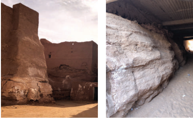
Figure 5: Tafza stone as a support of old building in the Ksar of Timimoun.
