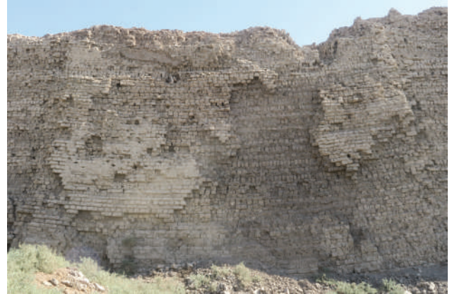
Figure 5: View of one of the wall sections nearby the eastern gate. The facing is damaged and shows layers of mud bricks on edge.
