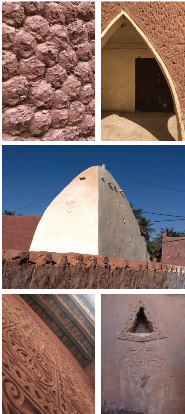
Figure 10: Exterior earthen and lime plastering (on top). Decoration techniques found in Timimoun (on bottom).
