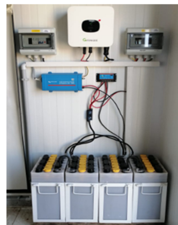
Fig. 15. Battery storing system.
