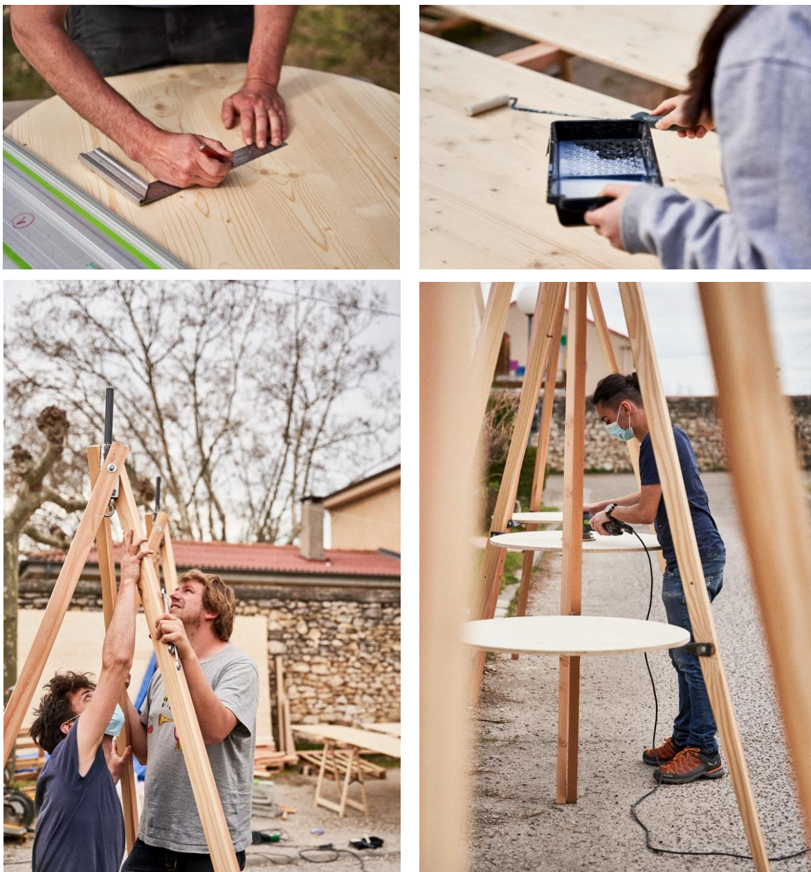
Figure 3. Photographs of the first week of construction in the retirement home, construction of totems in wooden cleats with the students Nîmes, 2021© Thomas Heydon.
