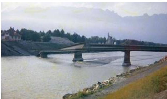
Fig. 7. The collapse of the bridge between Schaan and Buchs in the seventies was caused by gravel extraction from the river Rhine (photo by the authors).
