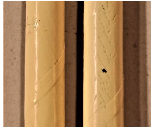
Figure 9 Unaged cable (left) and aged cable after breakdown (right). Note in the aged cable a degradation in the form of brand prints and a perforation resulting from the breakdown.
