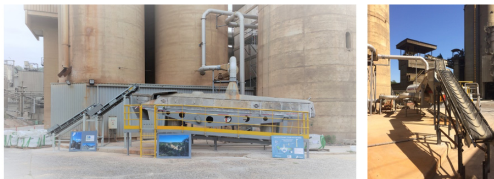
Figure 5. Fluidized bed at the LafargeHolcim Val d'Azergues cement plant.
