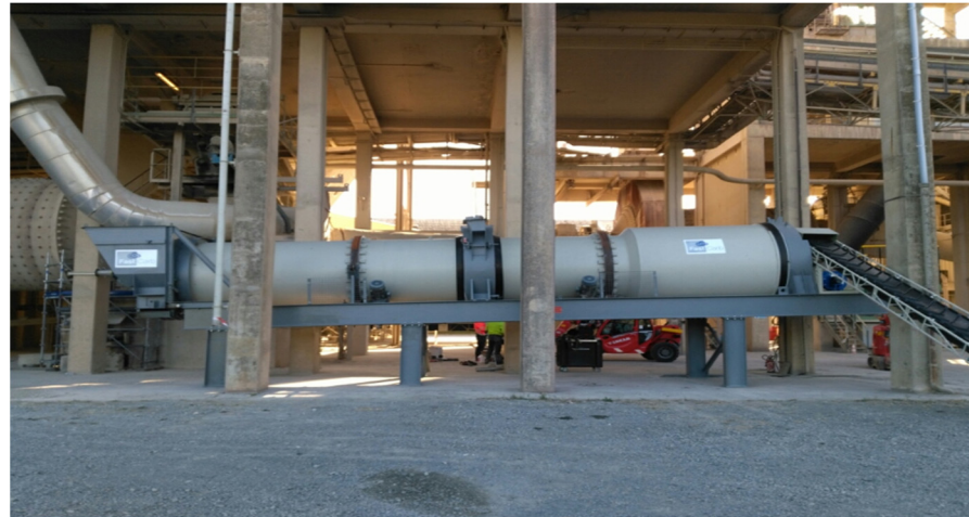
Figure 4. Rotating drum at the Vicat Créchy cement plant.
