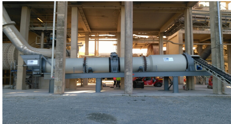
Figure 4. Rotating drum at the Vicat Créchy cement plant.
