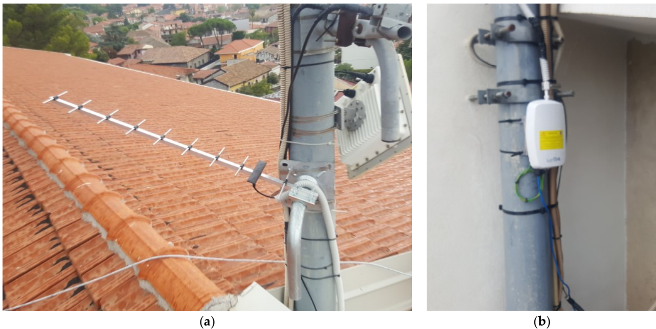
Figure 5. Layout of the gateway set-up on the roof top of Dusmet school in Nicolosi including a Yagi-type antenna pointing toward the Etna summit (a) and the Kerlink gateway at the bottom of the same mast connected to the antenna and to the power grid (b).
