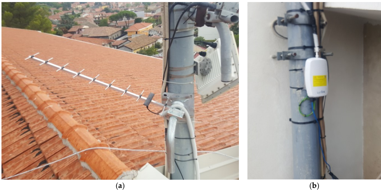
Figure 5. Layout of the gateway set-up on the roof top of Dusmet school in Nicolosi including a Yagi-type antenna pointing toward the Etna summit (a) and the Kerlink gateway at the bottom of the same mast connected to the antenna and to the power grid (b).
