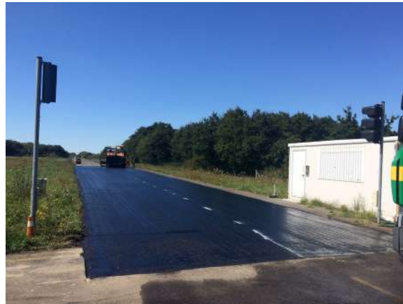
Figure 3.7: Laying of the tack coat (bitumen emulsion) prior laying of the VTAC 0/6.
