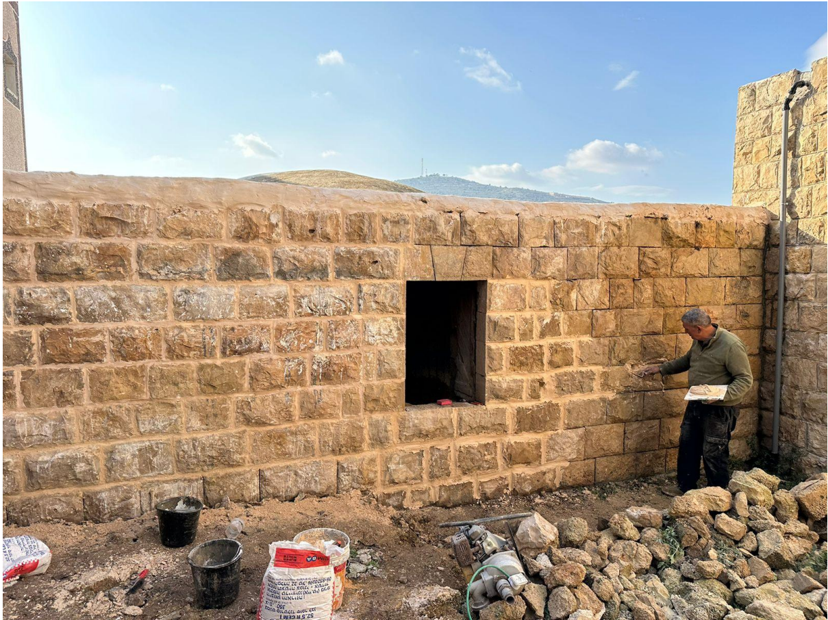
2. Yousef Iwaisi renovating the external walls of the family's traditional House (courtesy Mahdi Iwaisi 2024).
