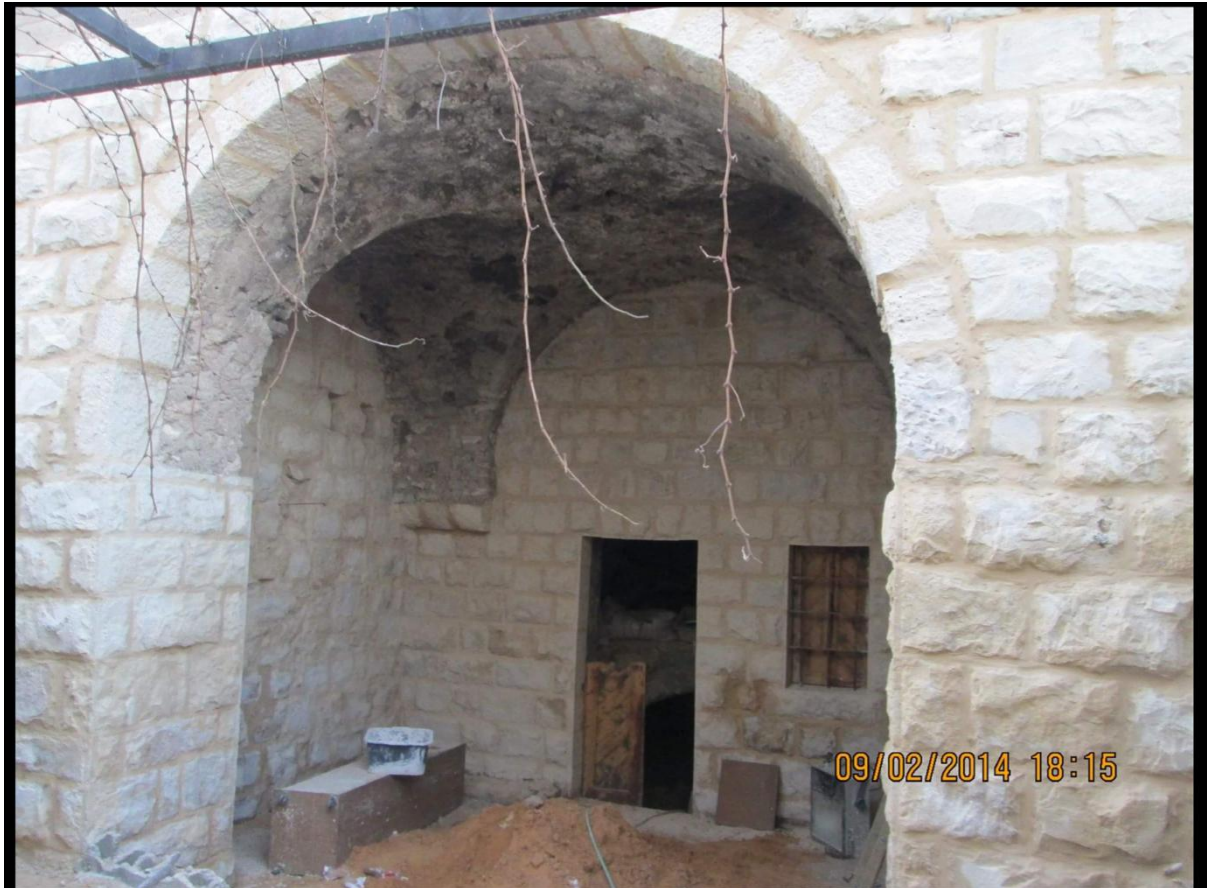
1. 1 st stage of Renovating Mazen Iwaisi's Traditional House in 2014 (courtesy Monther Iwaisi 2014).
