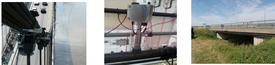
Figure 2. a) cable-monitoring b) water-network monitoring c) deck monitoring.
