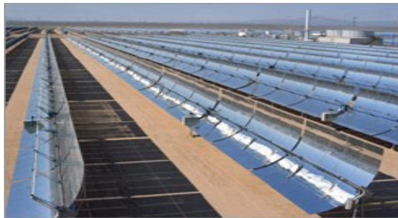
Figure 6. Parabolic Collector of the Power Plant.
